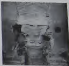
Fig. 143. S. Sisto Vecchio. Column base and shaft, seen from cloister wing (left) and printing press chamber.
